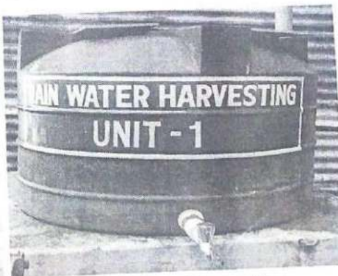
Rain Water Harvesting
